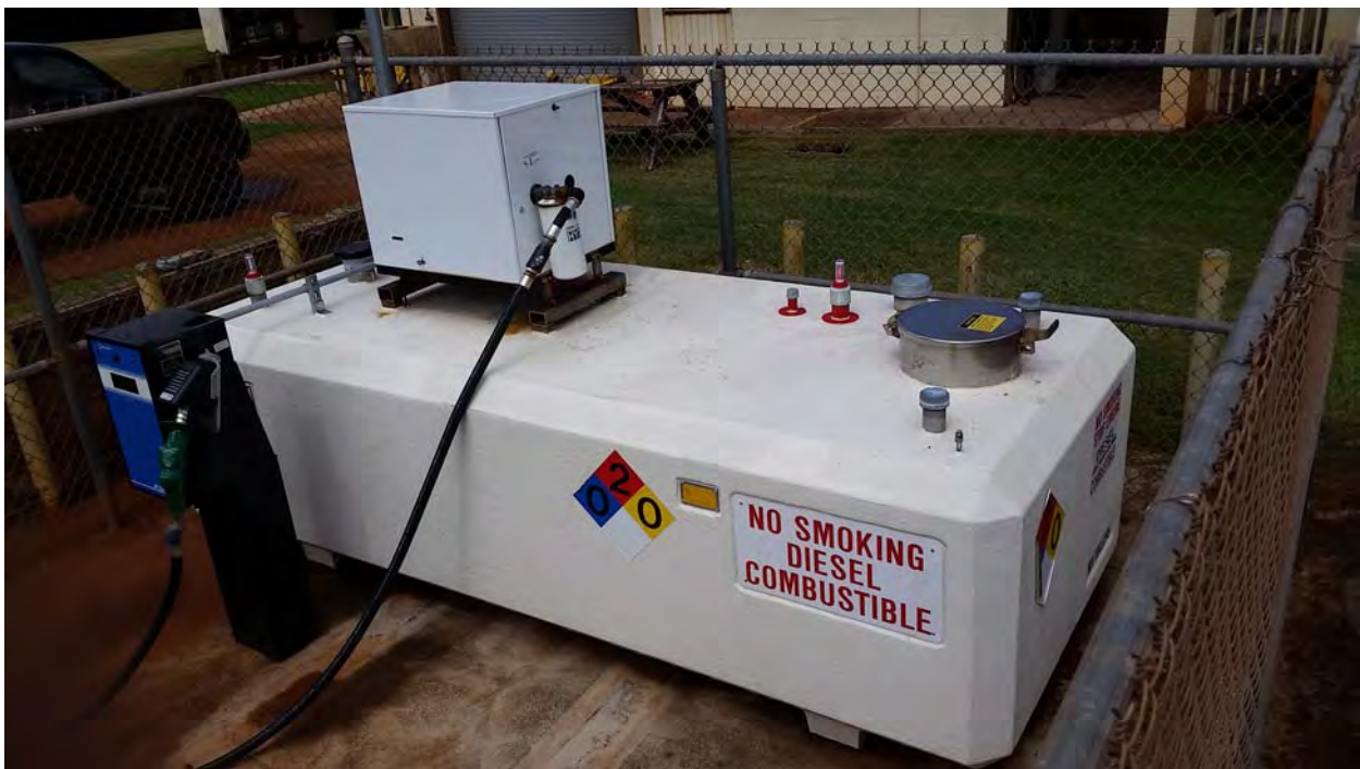
Ho'olehua Fire Station Fuel Tank
