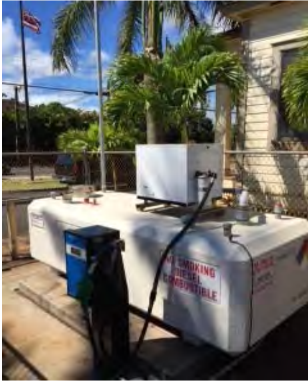
Paia Fire Station Fuel Tank
