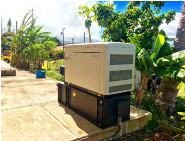
Lana'i Fire Station Generator
